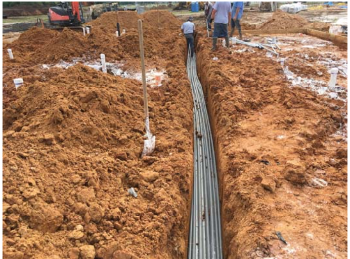
14. Underground electrical to home side elements
