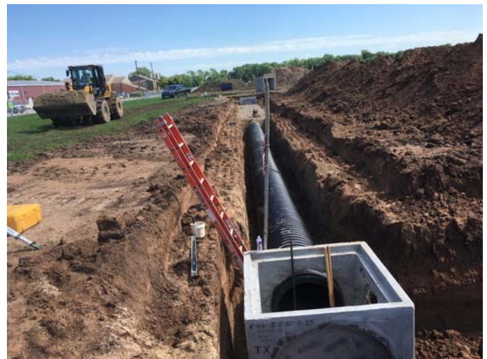
12. Storm sewer at home parking
