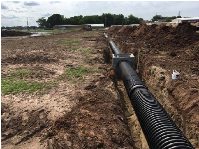
15. Storm sewer at home parking
