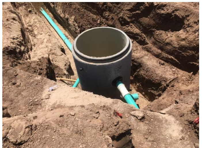
10. Sanitary manhole and piping at concessions
