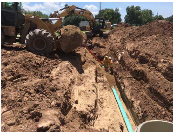
11. Sanitary sewer connections
